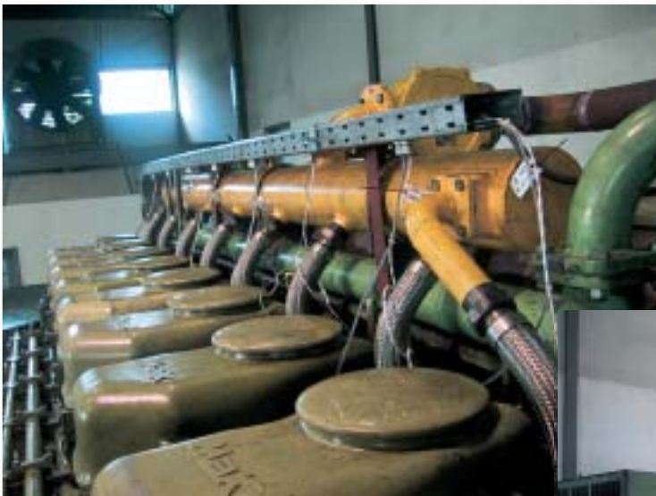
▲ Gas distribution pipe
