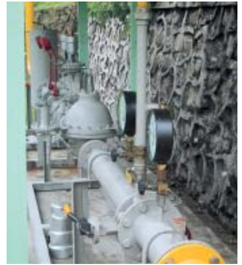
■ Main gas train
