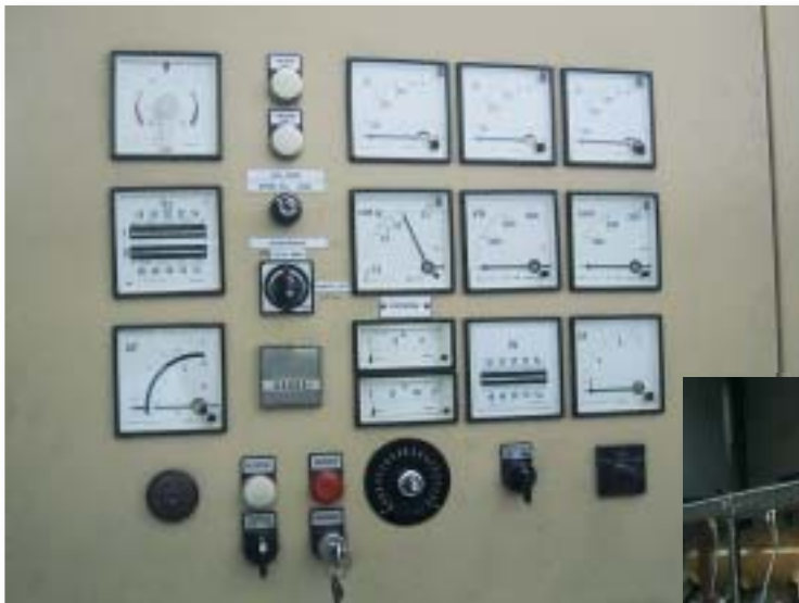
▲ Original switch board
